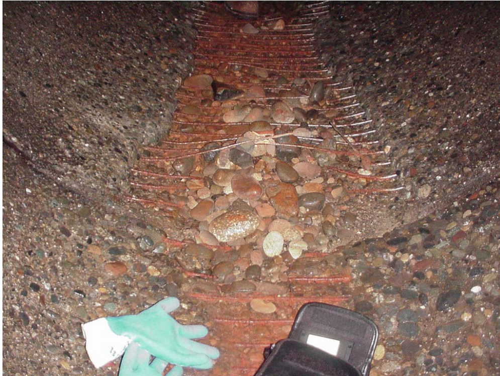
Figure 38. Interior structural damage to railroad culvert MP 28.24.
